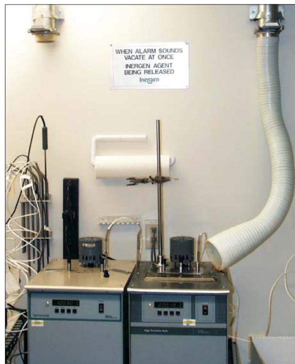
Figure 1 Ventilation system for removing oil vapors.
