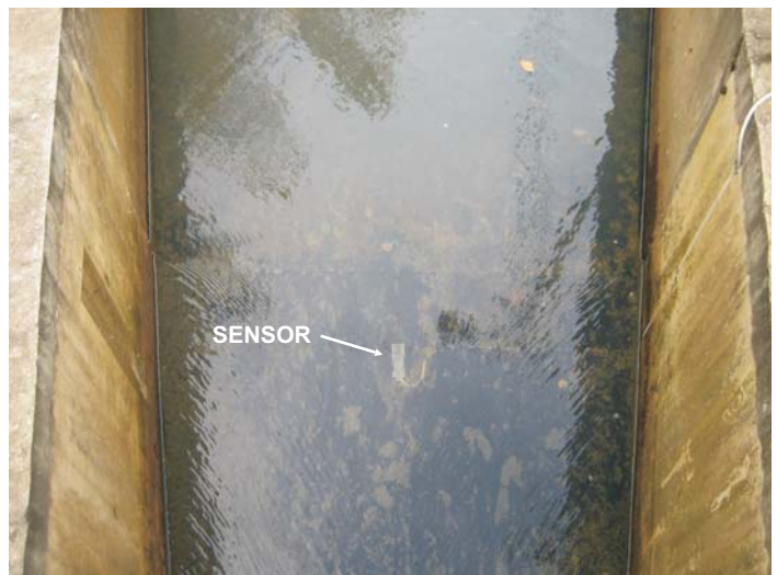
Stingray ultrasonic sensor installed in the approach section of a Parshall Flume
