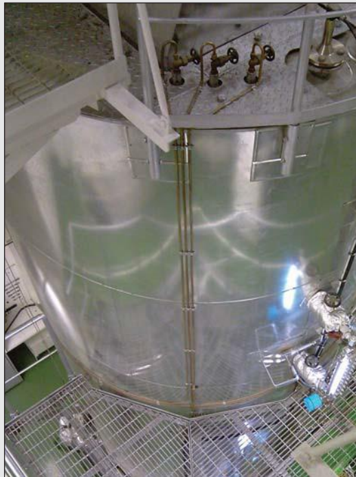
Marine Auxiliary Boiler
