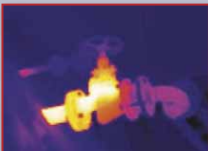
A hot-water valve, shot in the dark
