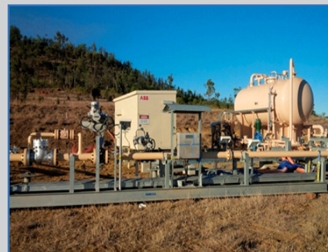
► Coal Seam well-head with water separator
