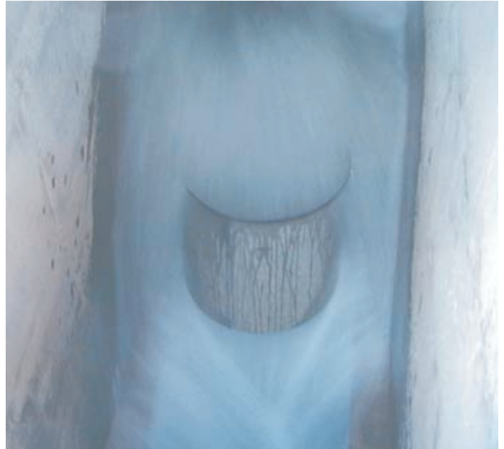
Fly Creek Pump Station
